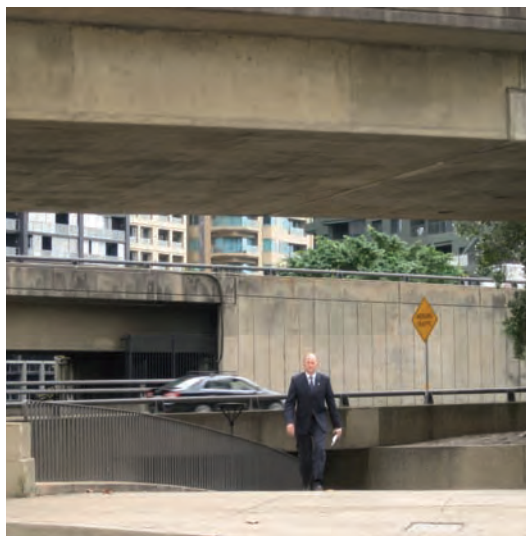
The Kent Street underpass is where pedestrians are confronted with the mishaps of the traffic structure. People DO have to walk here because there is nowhere else to get across in the area.
