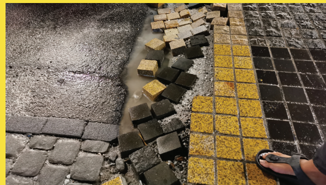
Picture 25: Temporary public works makes the surface unstable and unsafe, compromising walkability and public access.
